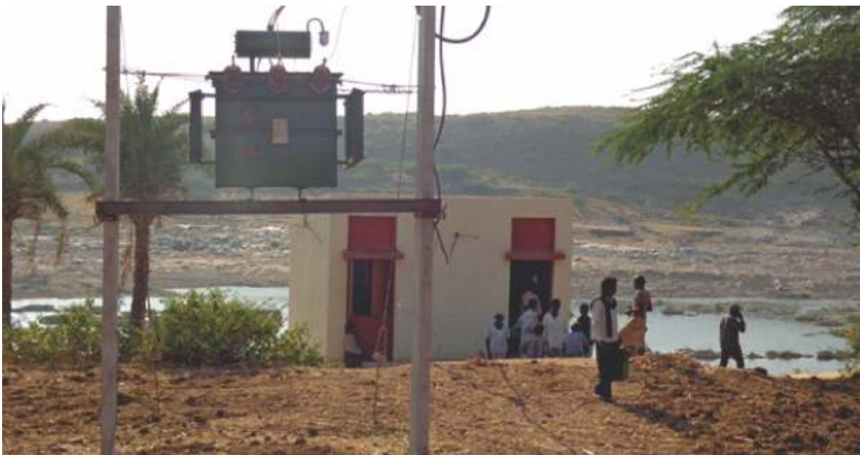
A pump house in Taluka Kushalgadh, District Banswara
